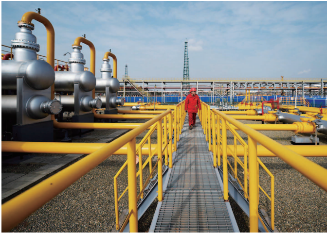
PetroChina Tower Southwest natural gas comprehensive utilization project
