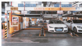
Parking lot Management
