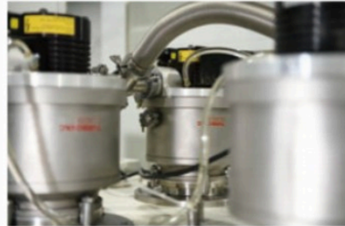
Vacuum System consists of mechanical fore pumps and molecular vacuum pumps.
