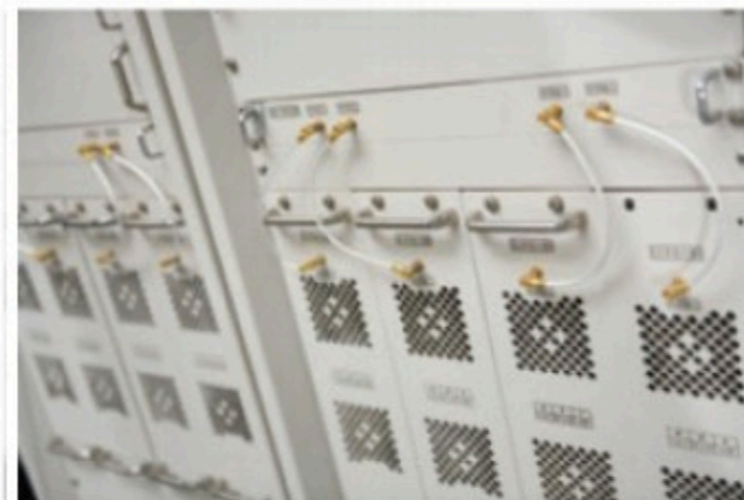
High-frequency Power Supply System provides strong RF electric field to accelerate proton beam.
