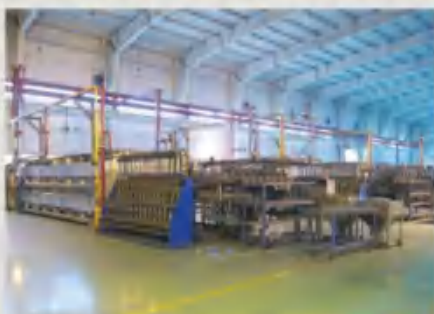
氢气还原设备 Hydrogen reduction equipment
