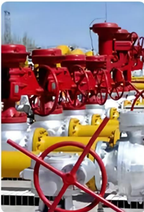
Oil pipeline system
