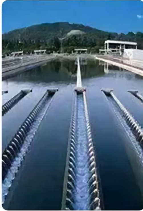
Tap water plant
