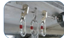
3S Horizontal Lifeline System fixed on the roof by bolts.
