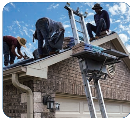
Roof Photovoltaic Installation
