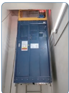
Environmental Protection Plant
