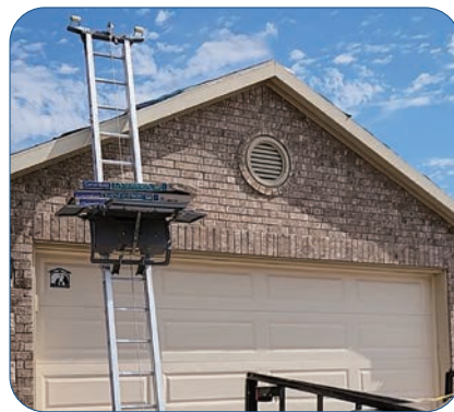
Roof Photovoltaic Installation
