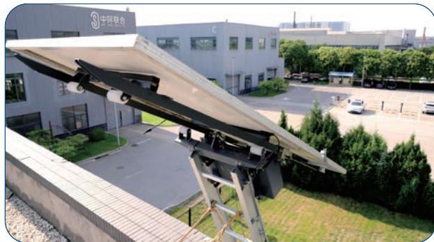
Building Roof Photovoltaic Installation
