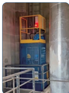
Environmental Protection Plant
