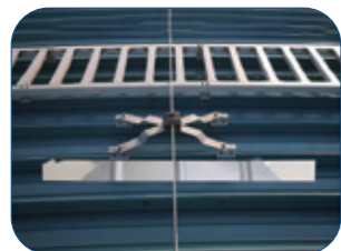
3S Horizontal Lifeline System fixed on color steel tile roof.
