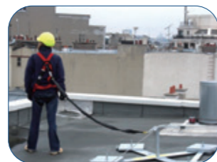
3S Horizontal Lifeline System attached to the counterweight.
