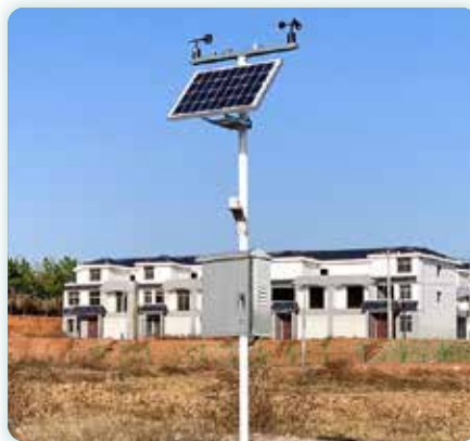
weather observation station
