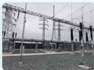
Intelligent inspection in substations
