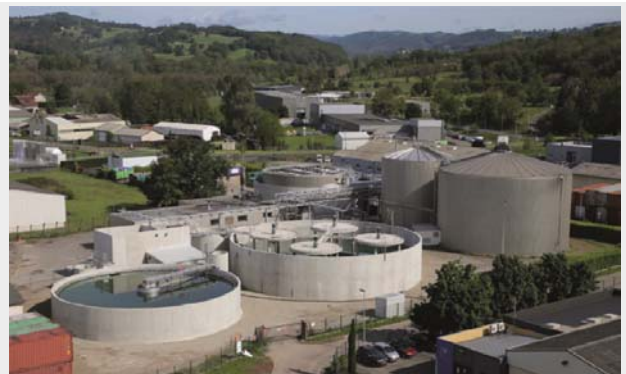
The new water treatment plant implemented in 2020 on the Biars site will increase the reliability of our discharges into the natural environment.
